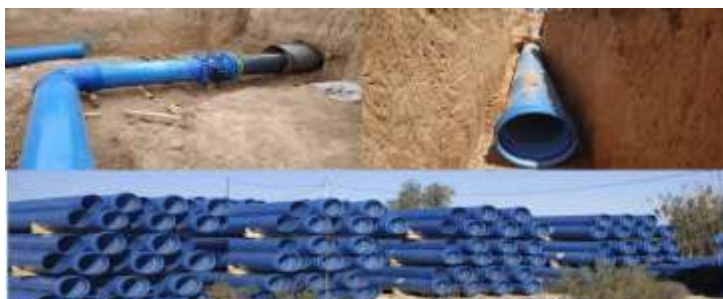
Figure - 2: Irrigation Pipelines – Egypt
